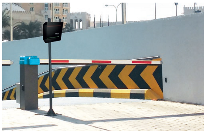
Parking Management: Comfortable access without waiting
